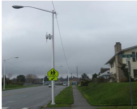
Figure 3: Wireless Access Point Mounted on Street Light
