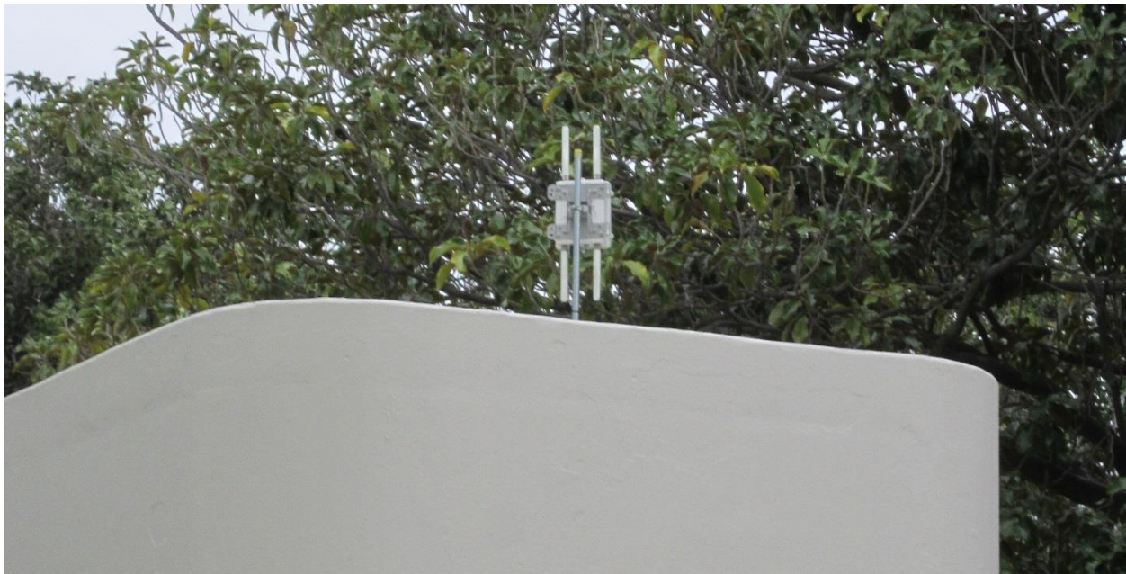
Figure 18: Wi-Fi Access Unit in Palo Alto
