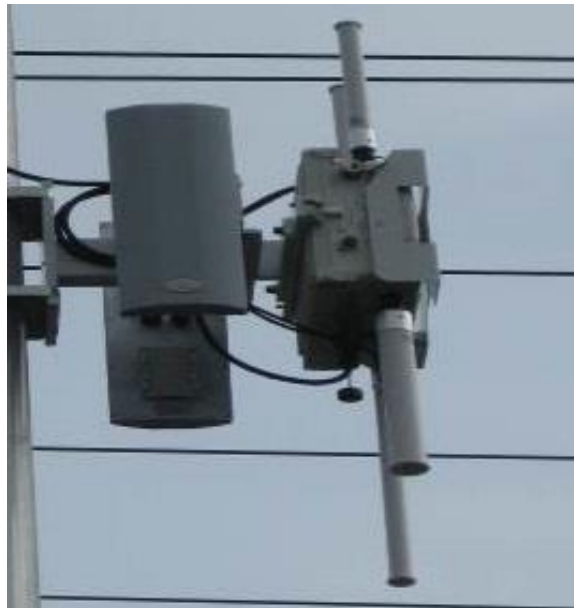
Figure 16: Typical Wireless Access Point Installation for Mesh System
