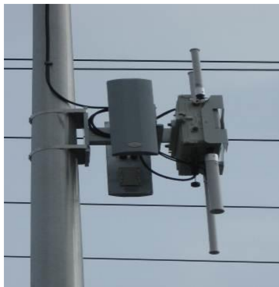
Figure 4: Wireless Access Point (Detail)
